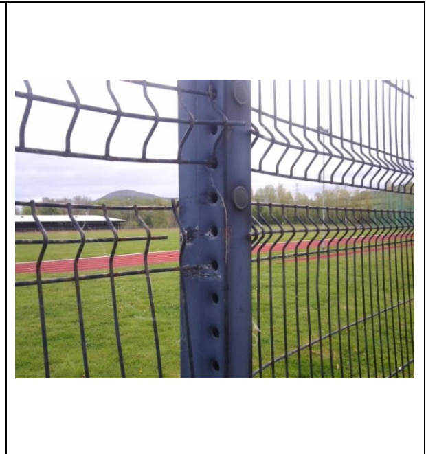
Damage to Mesh fencing
