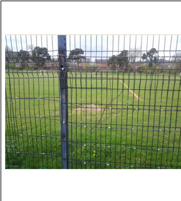
Damage to Mesh fencing
