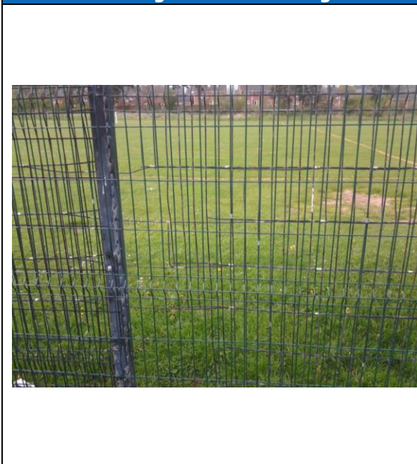
Damage to Mesh fencing
