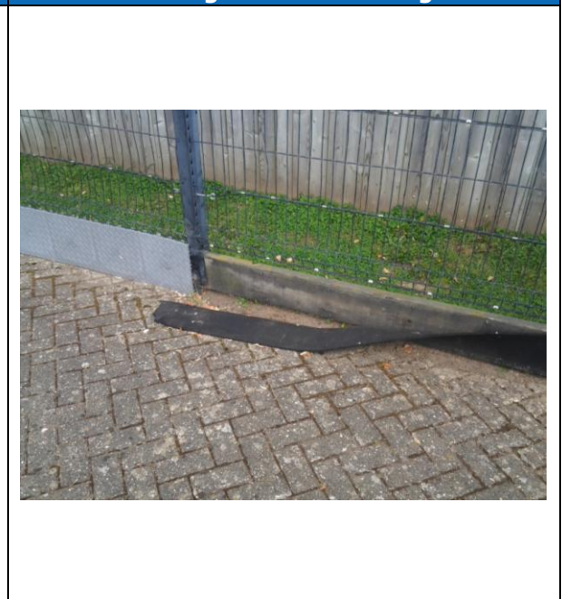
Rubber matting loose on boards.
